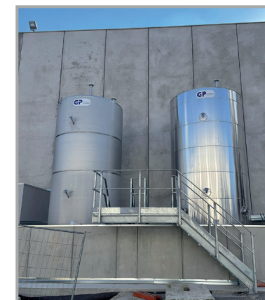
SERBATOI SU GAMBE DA 50 MC RISCALDATI E COIBENTATI PER OLII PLASTIFICANTI 50 M 3 HEATED AND INSULATED TANKS ON LEGS FOR PLASTICISER OILS
