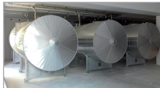
CISTERNE DA 20 MC RISCALDATE E COIBENTATE PER OLII PLASTIFICANTI 20 M 3 HEATED AND INSULATED CISTERN FOR PLASTICISER OILS
